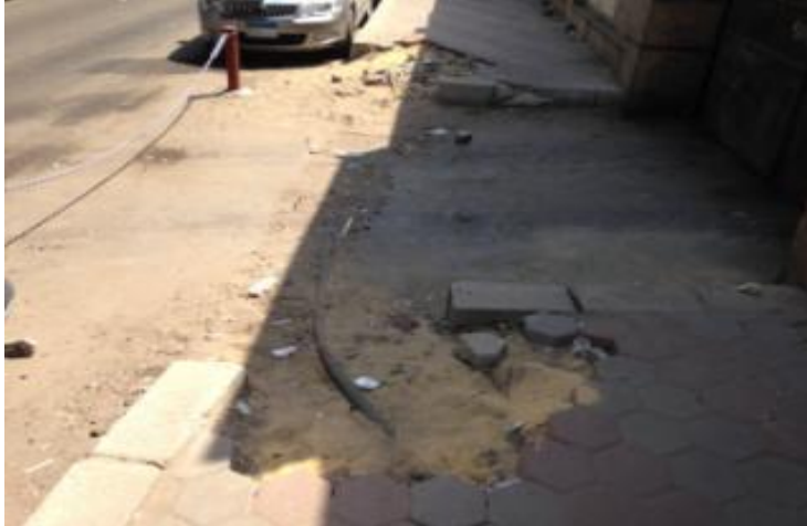
Figure 42: Road Conditions poor
